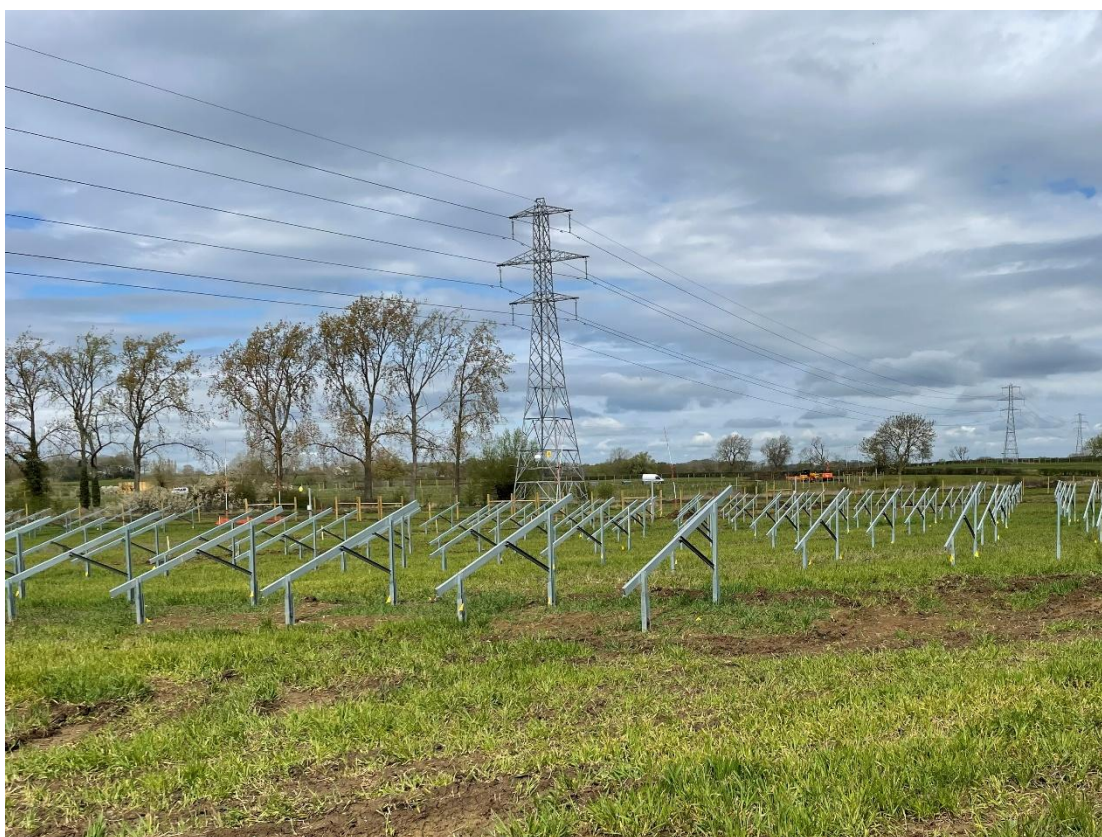
Plate 3-2 Example of Solar PV Mounting Structures (Source: Low Carbon)
