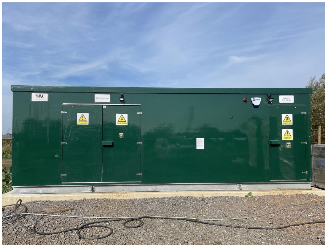
Plate 3-3 Example of a Power Conversion Unit housed within a container (Source: Low Carbon)
