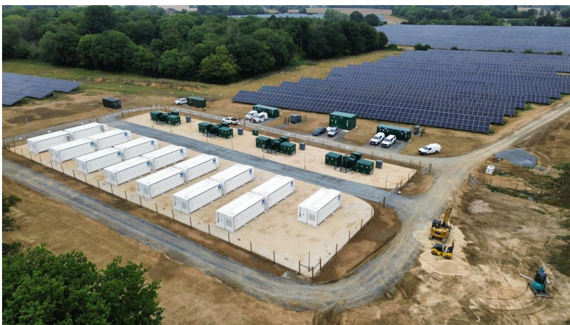
Plate 3-4 Example of BESS units grouped within a compound (Source: Low Carbon)
